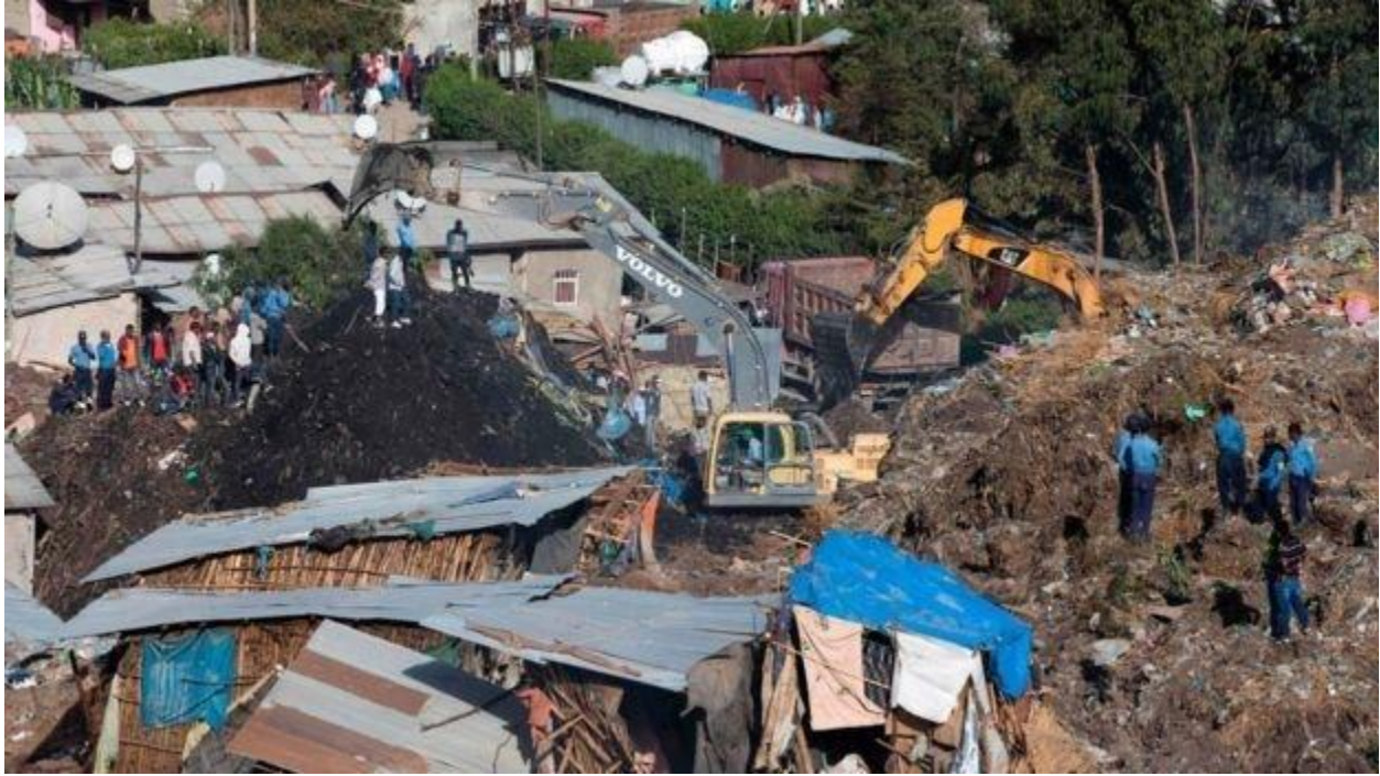
Landslide incident in Oromia region, 29 May 2018
