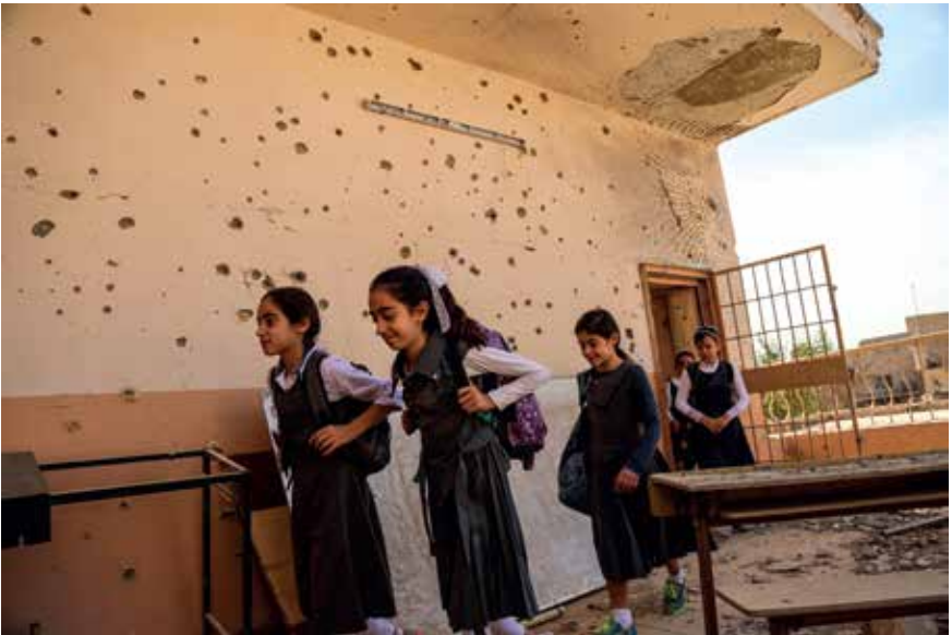
Damage from conflict is clearly visible at a school/ Ramadi, Anbar Governorate , Iraq/ Wathiq Khuzaie
