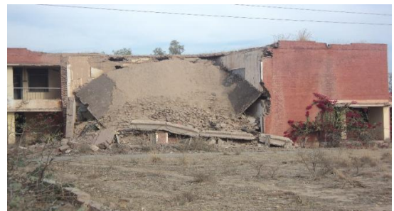
Credit: UNOPS Infrastructure damage in Bara. The inter-cluster assessment team to Bara found at least five schools totally damaged.
