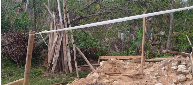
Photo: The home owner has salvaged usable timber and other materials. However, the salvaged timber is often old, and has some damage from water, insects and previous construction markings
