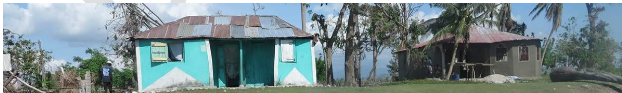
Photo: People are rebuilding wherever possible. The building pictured here has a roof repaired with a combination of salvaged and new corrugated iron
